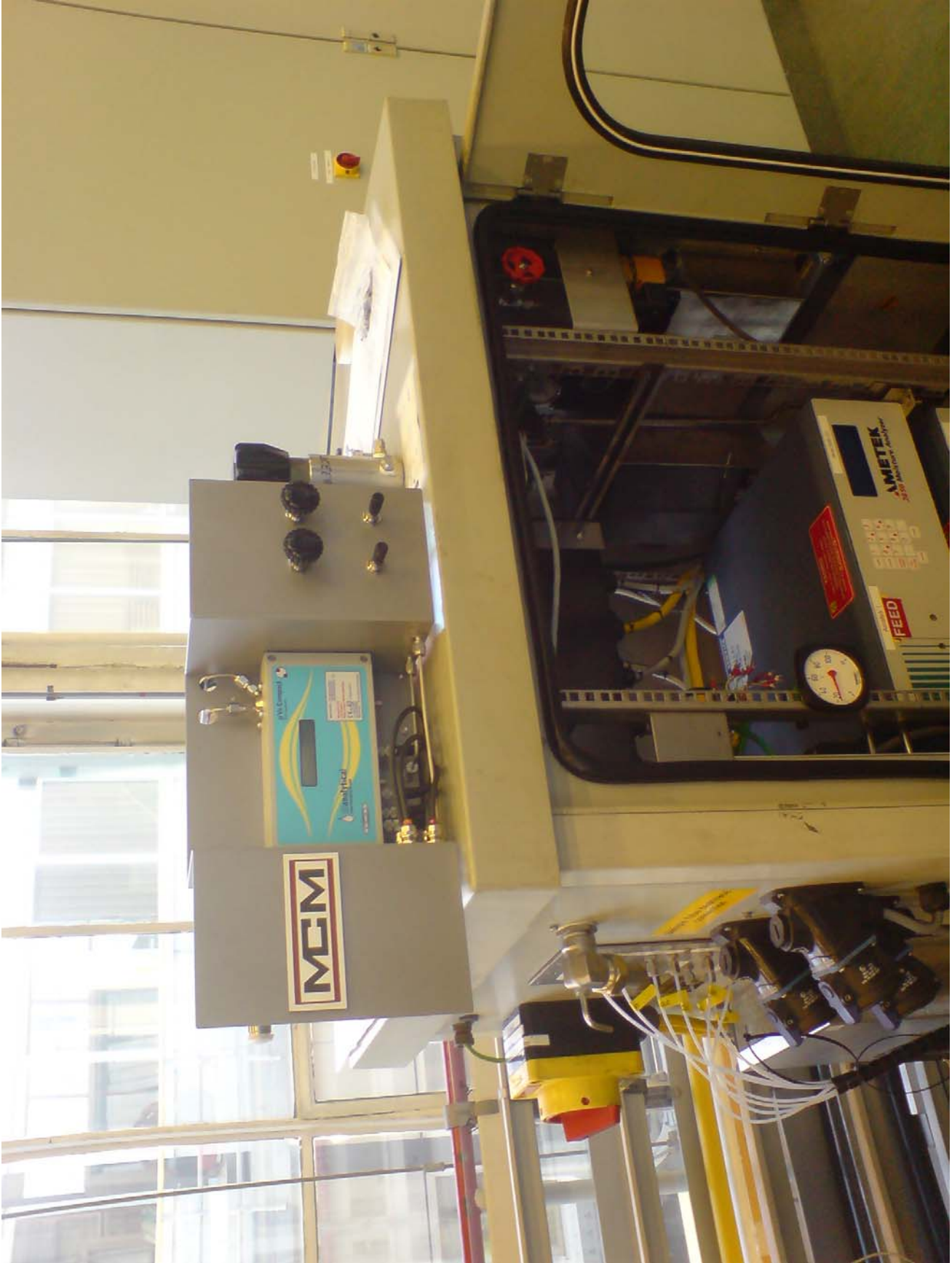
Figure 3 - The mobile analyser cabinet (MAC) used for water capacity test runs, with the MCM Auto-Zero transmitter unit prior to its installation (Note the MAC's PTFE sample inlets).
